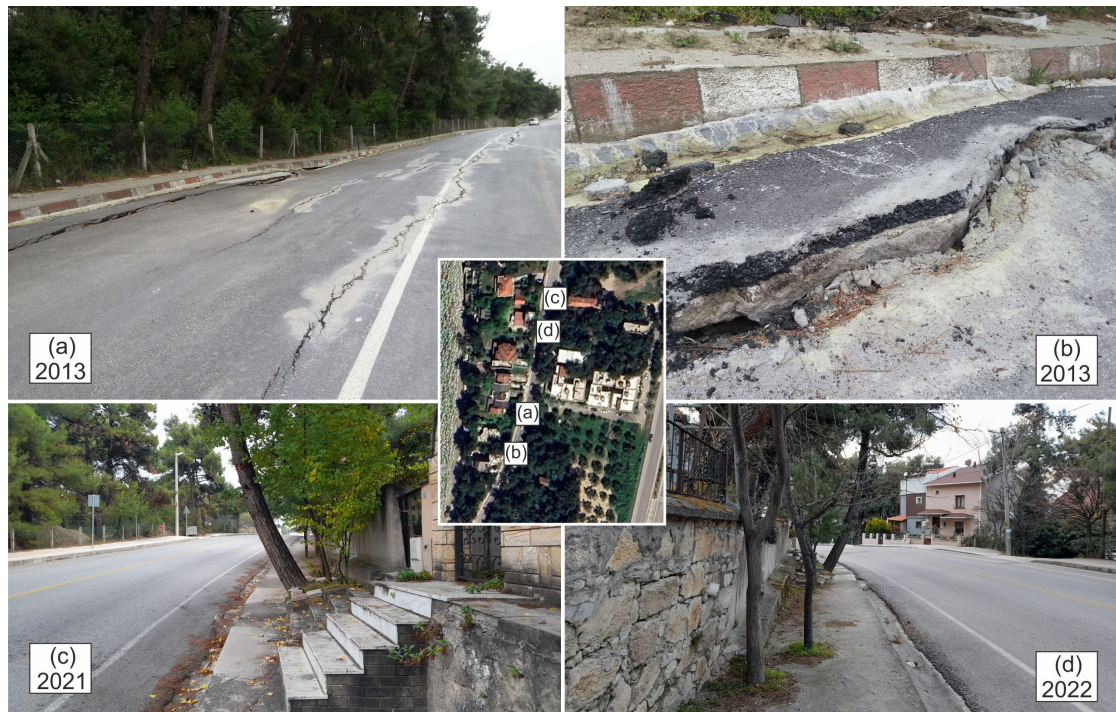
Figure 6. Images showing damage from the 2013 landslide and subsequent reactivation in 2021 and 2022, with their locations marked on the provided aerial photograph.
