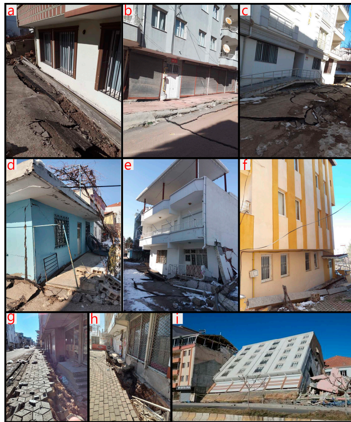
Figure 3. Examples of ground-based damage (a–f): undulations and collapses in the ground; (g,h): liquefaction; (i): inadequate soil–foundation connection.
