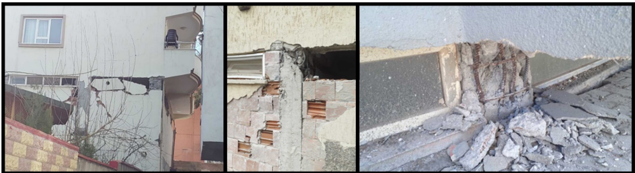
Figure 14. Examples of damage caused by short columns.
