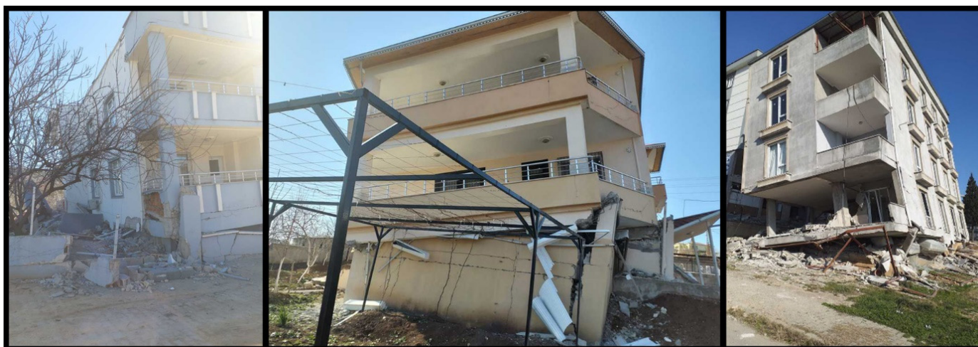
Figure 4. Examples of out-of-plane damage in columns.
