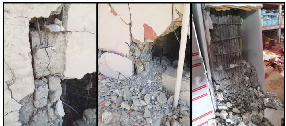
Figure 12. Examples of damage resulting from poor reinforcement workmanship.
