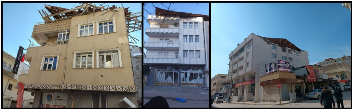
Figure 28. Samples of roof gable wall failure and collapsed roof.
