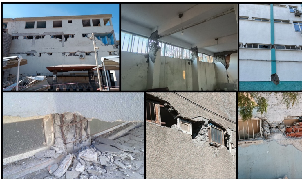
Figure 13. Examples of short column damage.
