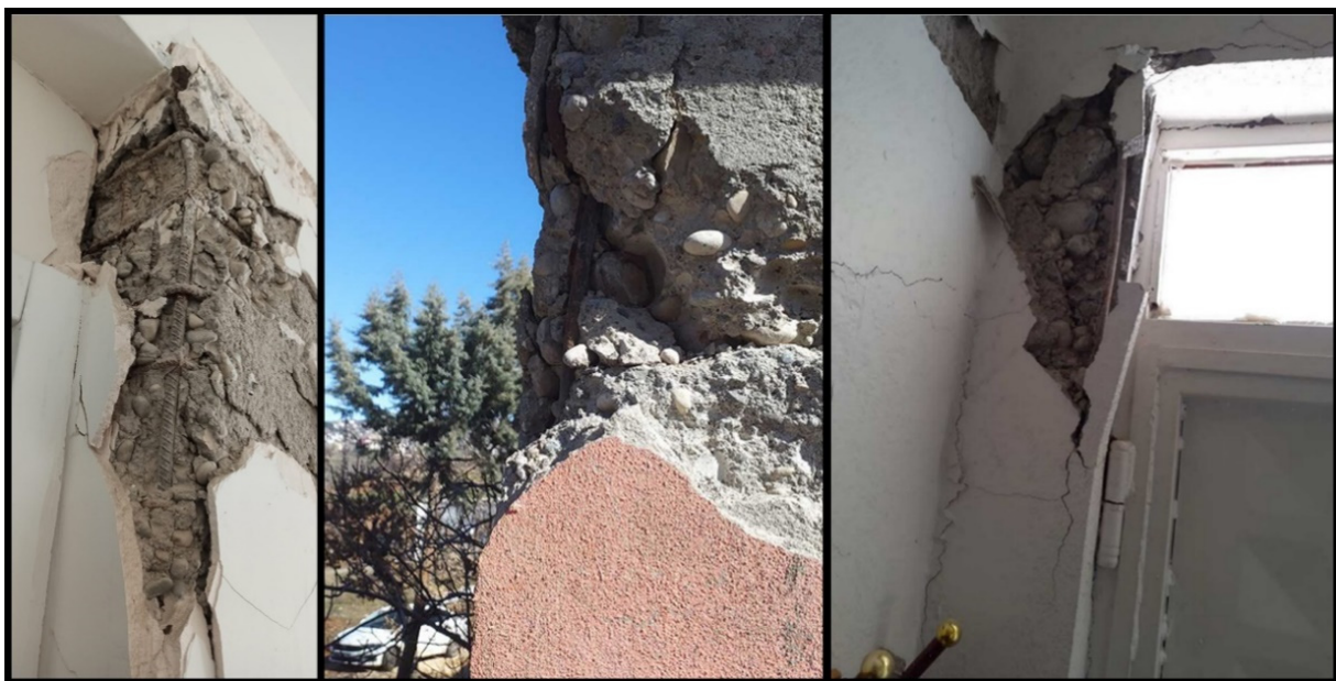
Figure 29. Examples of structural damage resulting from improper aggregate granulometry.
