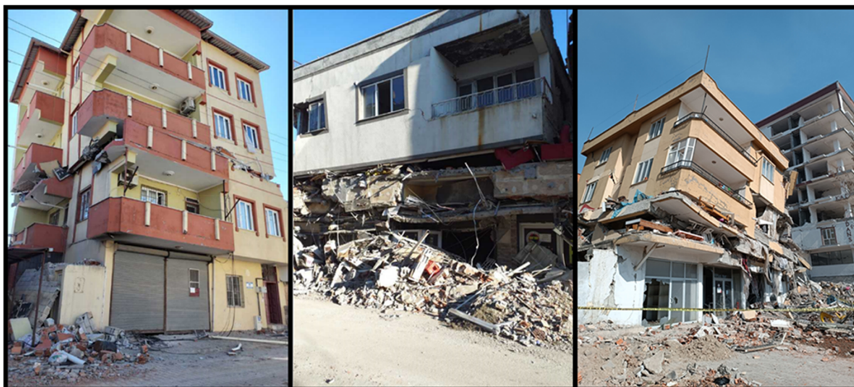
Figure 9. Samples of weak story damage.
