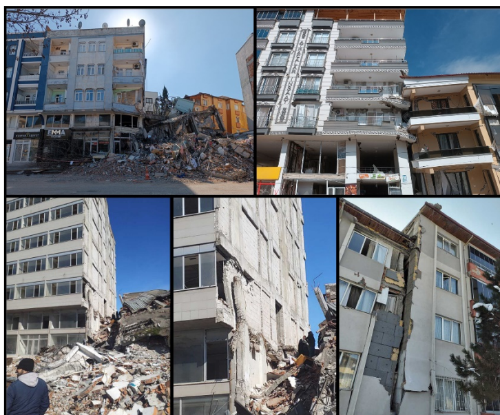
Figure 21. Structural failures caused by the pounding effect.
