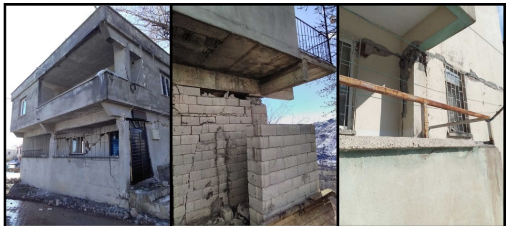
Figure 20. Examples of the plastic hinge damage due to the cantilever beam effect.
