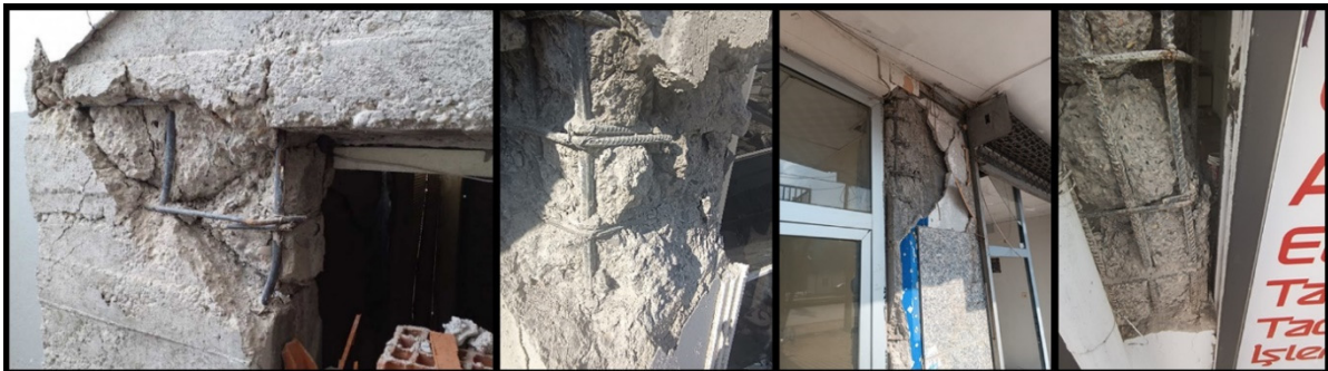
Figure 24. Structural failures caused by application fault of stirrups.
