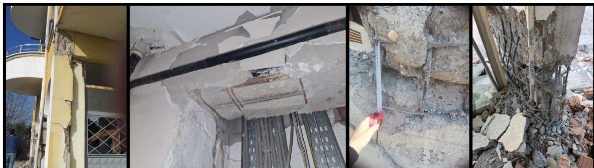
Figure 32. Structural failures caused by insufficient transverse reinforcement.
