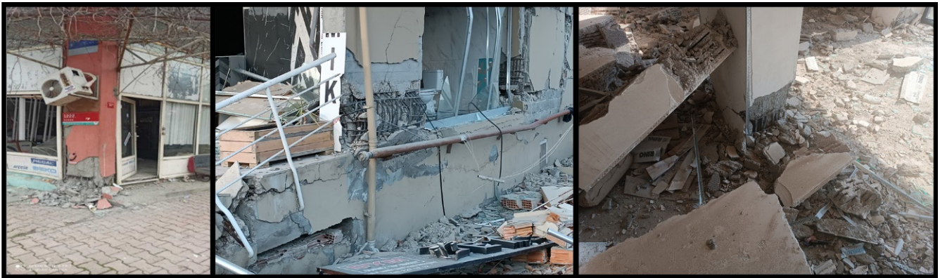
Figure 18. Examples of the plastic hinge damage at the lower end of the column.
