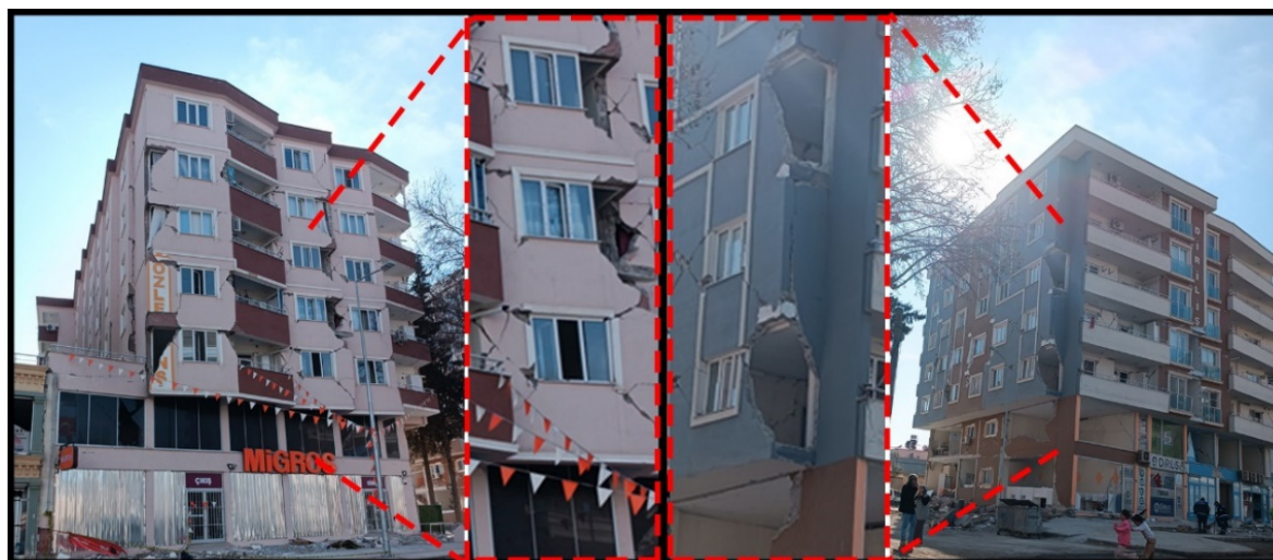
Figure 33. Examples of the structural damage caused by heavy overhangs.
