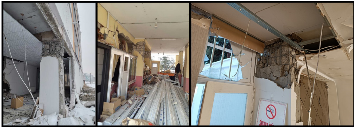
Figure 23. Structural failures caused by the crushing of core concrete in columns.
