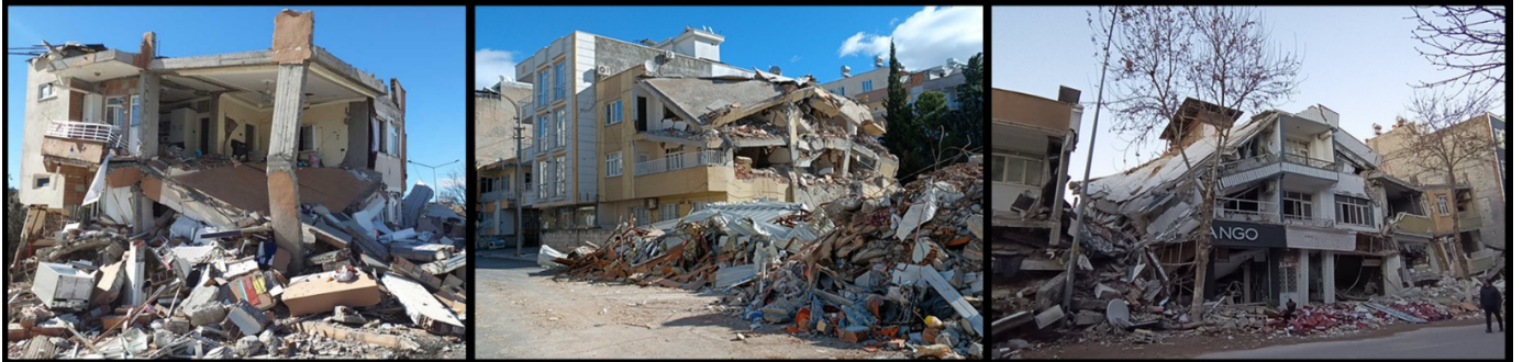
Figure 15. Damage caused by inadequate slab–beam–column connection.
