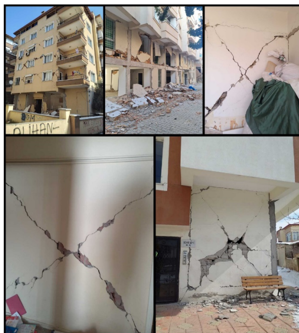
Figure 14. Examples of infill wall damage because of the Kahramanmaraş earthquakes.
