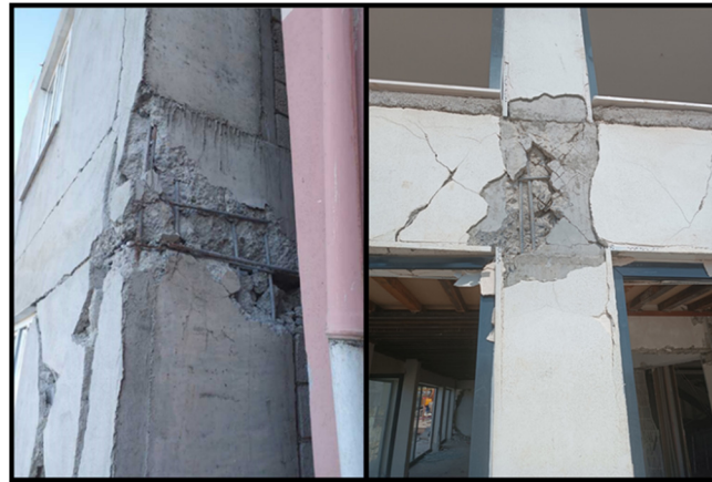
Figure 26. RC building damage caused by insufficient reinforcement in the column–beam joint.
