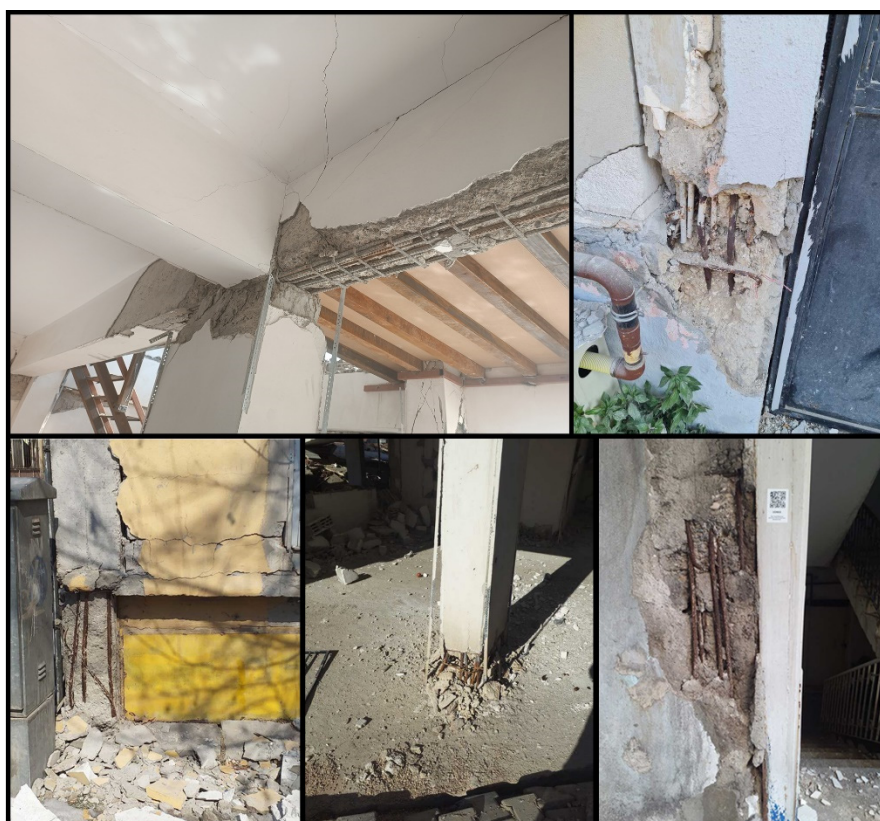
Figure 22. Examples of buildings with insufficient concrete cover.
