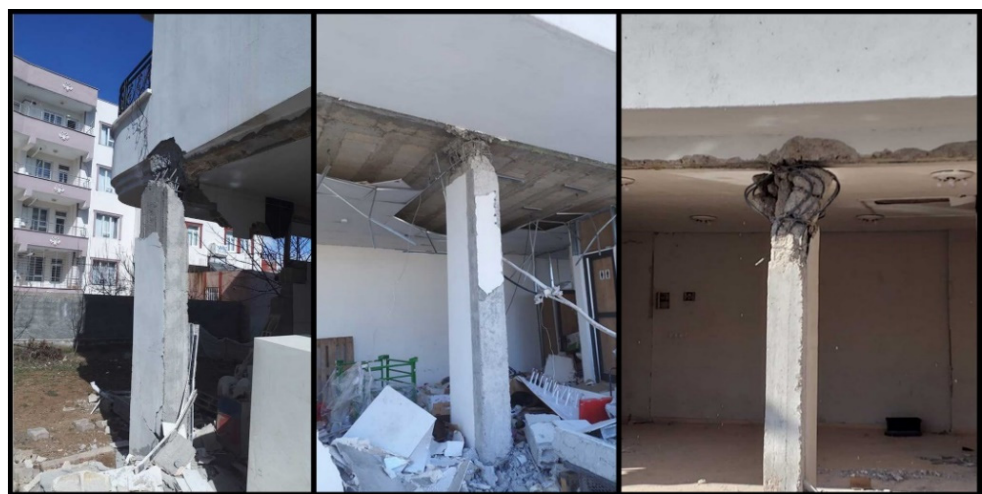
Figure 19. Examples of the plastic hinge damage at the upper end of the column.
