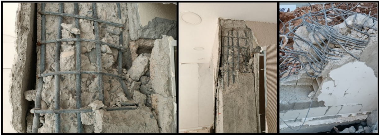
Figure 30. Examples of damaged structures using flat reinforcement.
