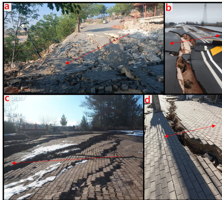
Figure 6. Ground-related damage after the earthquakes; (a,c) lateral spread towards a free face; (b,d) lateral spread down gentle slopes.
