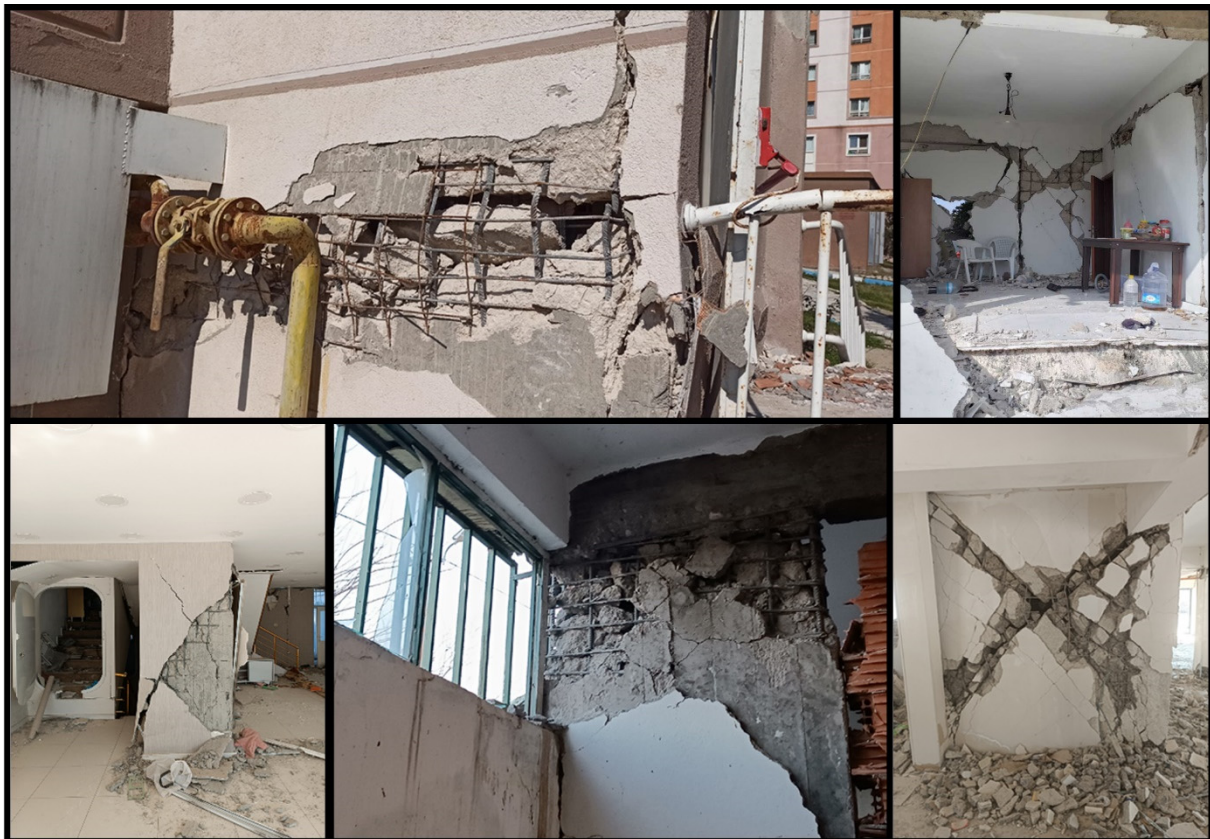
Figure 16. RC shear wall damages.
