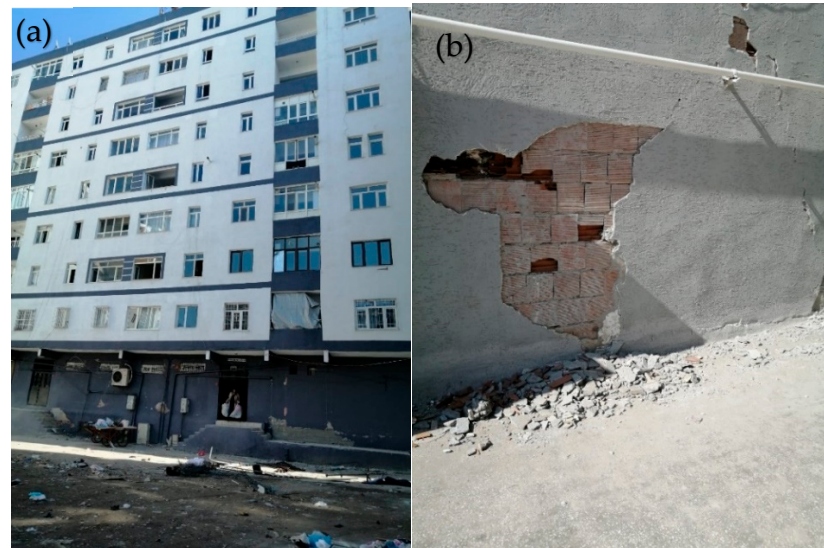
Figure 5. A building that sustained severe structural damage as a result of seismic activity: Photographs (a,b) show the Güçlü Apartment in the Bağlar district.
